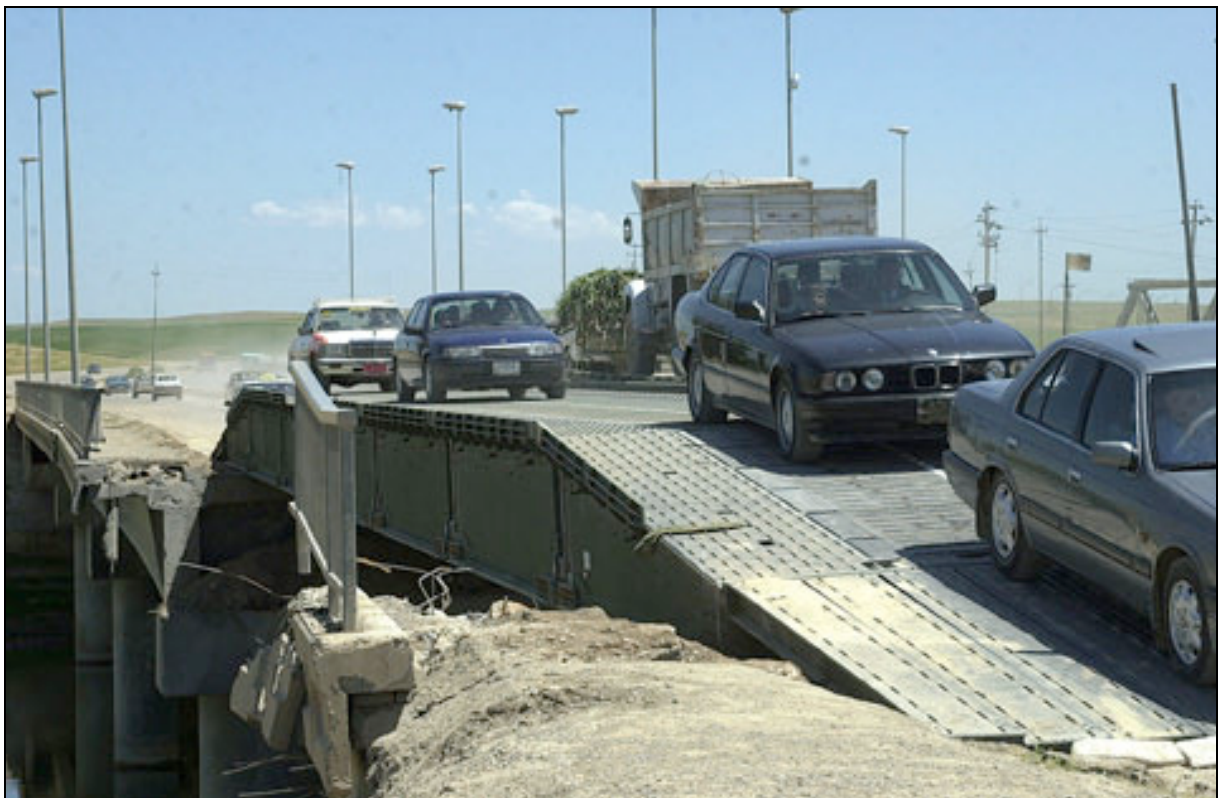
The DSB spanning the gap on a main highway in northern Iraq
